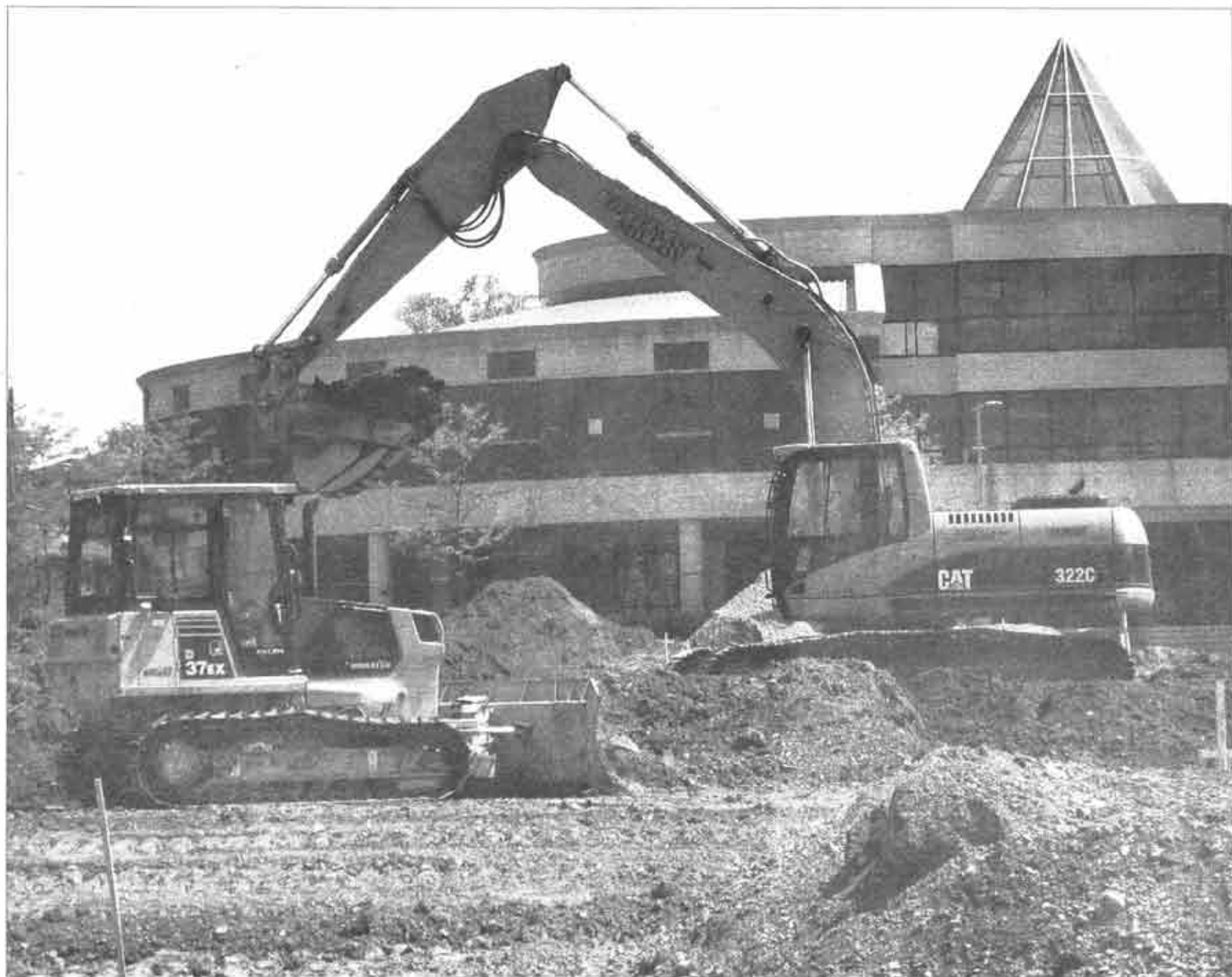
CONSTRUCTION ZONE - Willison Field gets all ripped up as it undergoes the first phase of its transformation into Alumni Field for Sept.
