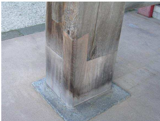
Figure 7 A new timber component was used to partially replace a rotten column with traditional carpentry
