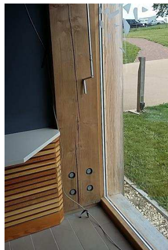
Figure 6 Vertical cracks occur in a column
