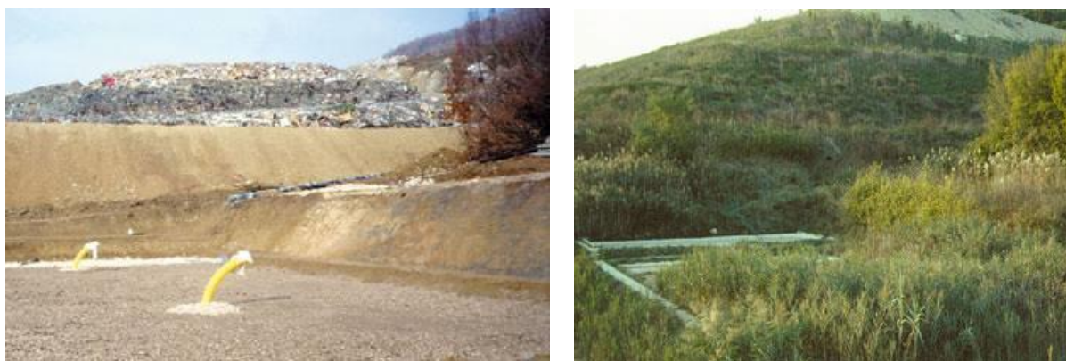
Figure 11: Constructed wetland Dragonja. (left) CW Dragonja in the phase of construction. (right) First cell of CW Dragonja
