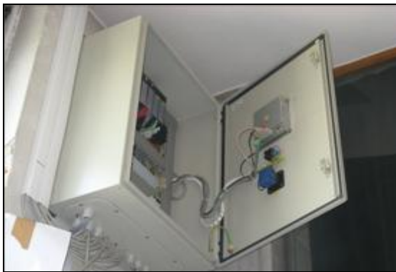
Fig 18: Building management system, hardware
