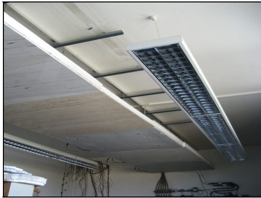
Fig 13: Heating and cooling panels
