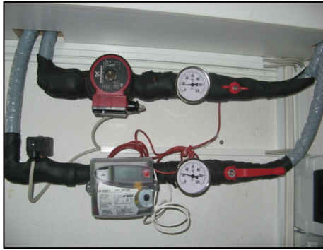
Fig 25: Ultrasonic compact heat and cooling meter
