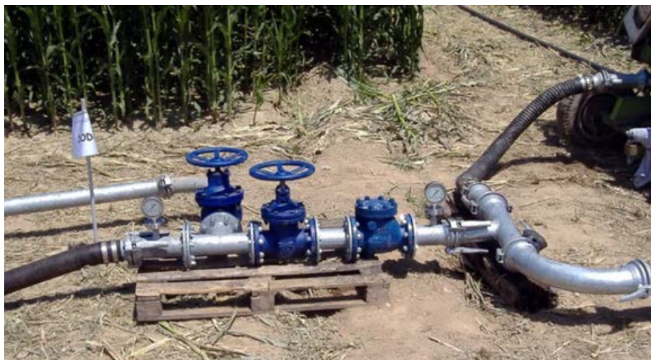
Figure 63: Membrane pump and injection system (Bassanino et al. 2008)
