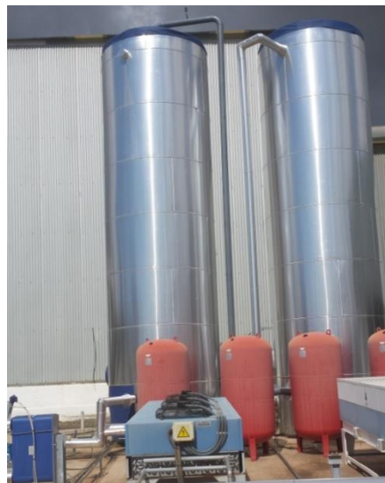
Figure 3. Thermal storage tanks installed at PSA
