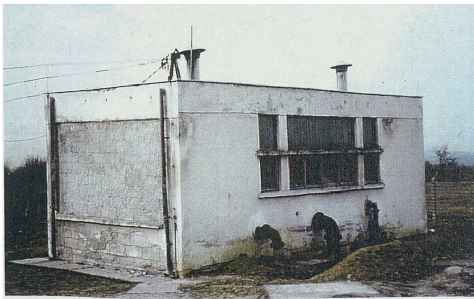
↕ The pumping station in Toplića
