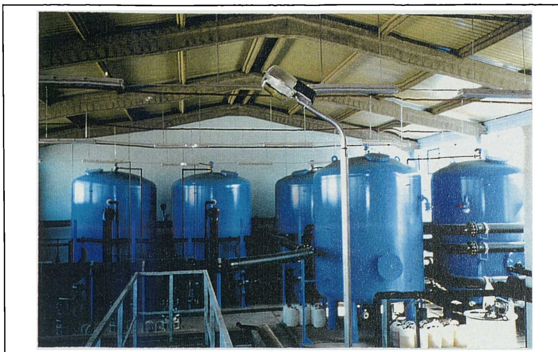
Figure 9.2: The water treatment plant in Gradačac (Source: Author)
