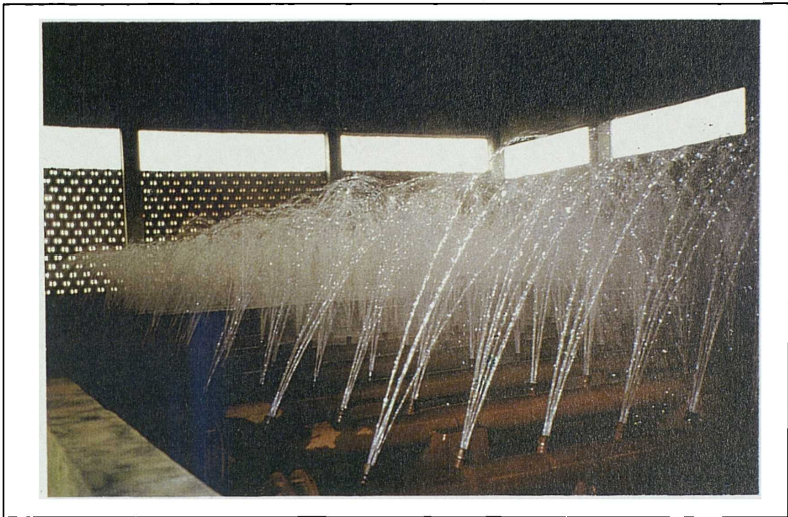
Figure 8.7: The Tuzla Water Supply's sprinkler aeration plant (Source: Author)
