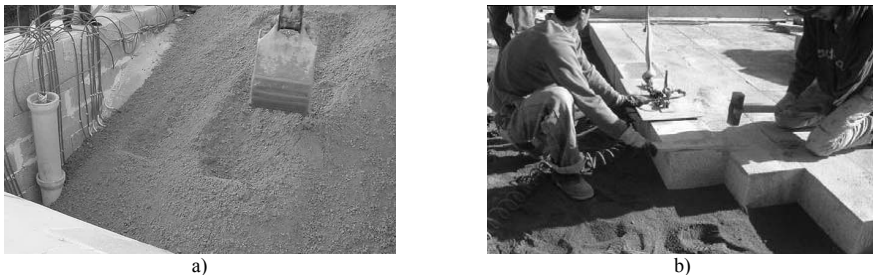
Figure 4 : Vila Fria bridge structure – (a) backfill material and (b) granite stone pavement
