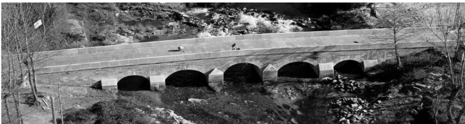
Figure 5: The new Vila Fria Bridge. Aerial view. Courtesy of Prof. F. Piqueiro and Foto Engenho ©.
