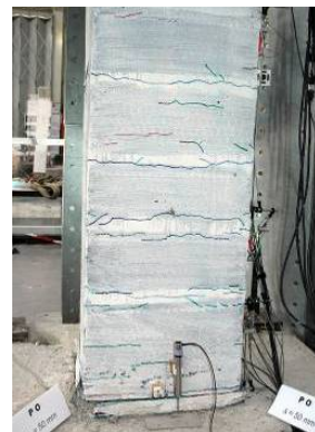
b) Final damage – south
