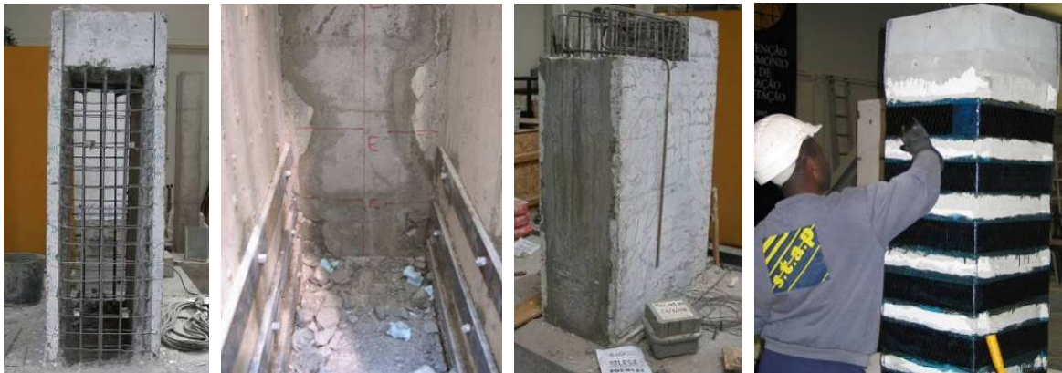
Figure 7 Hollow piers before and after the shear retrofitting with inside steel bars and outside CFRP sheet.
