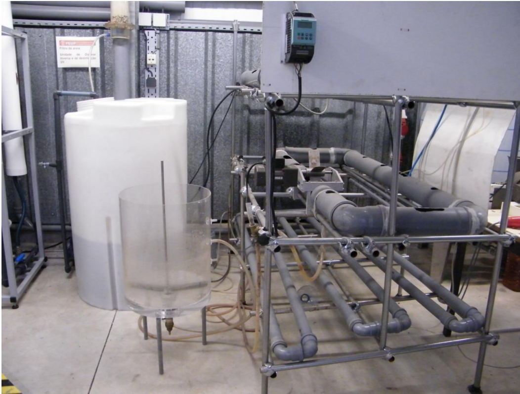
Figure 3.1 Pilot installation of the tubular closed-loop PFRR with feed tank and the secondary settler.
