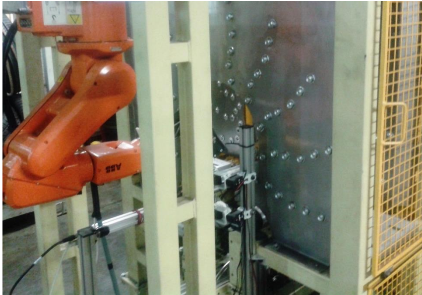
Figure 4.5 - Prototype installed at the manufacturing plant
