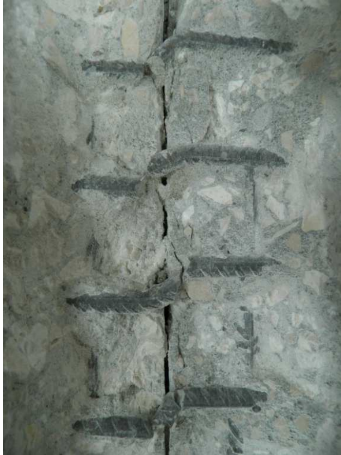
Figure 2-16 – Outlook of the reinforcement, after the removal of the concrete cover, of an interface subjected to a low amplitude cyclic loading.
