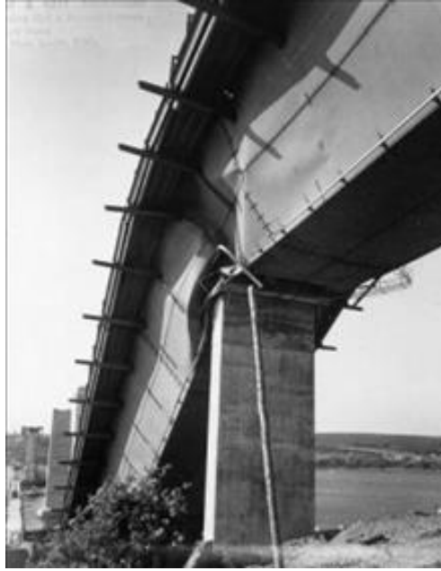
Fig. 2.21 – Colapso da Milford Haven Bridge (Stephen Cantrell et al)
