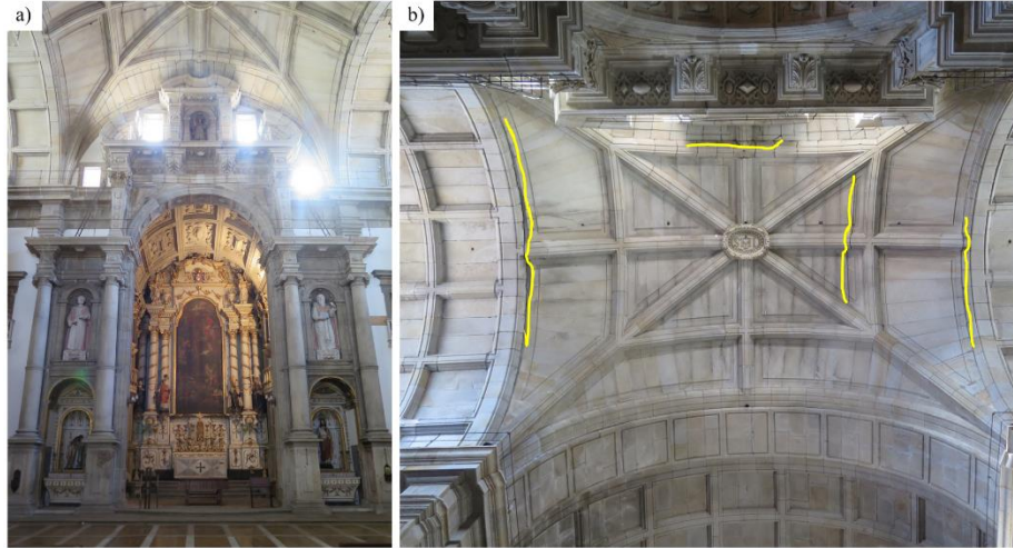
Figure 50. Altar-Mor of the São Lourenço Church: a) general view and b) main cracks occurrences.
