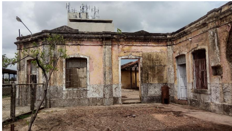
Figure 5. Material degradation by environmental action.
