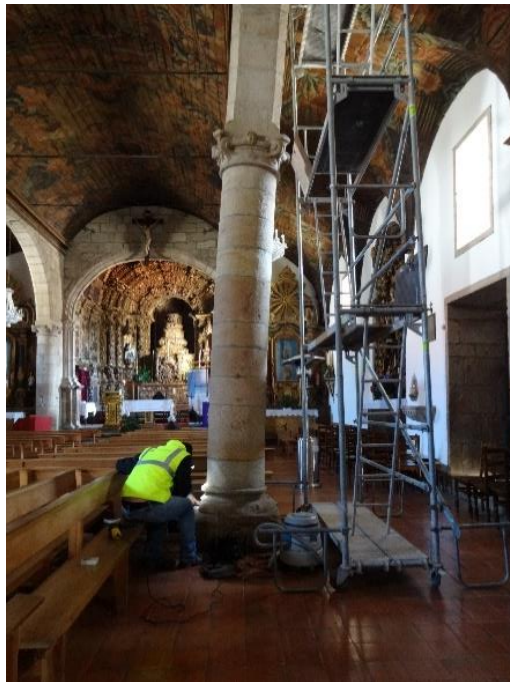
Figure 72. Photograph of column 2, evidencing its inclination.
