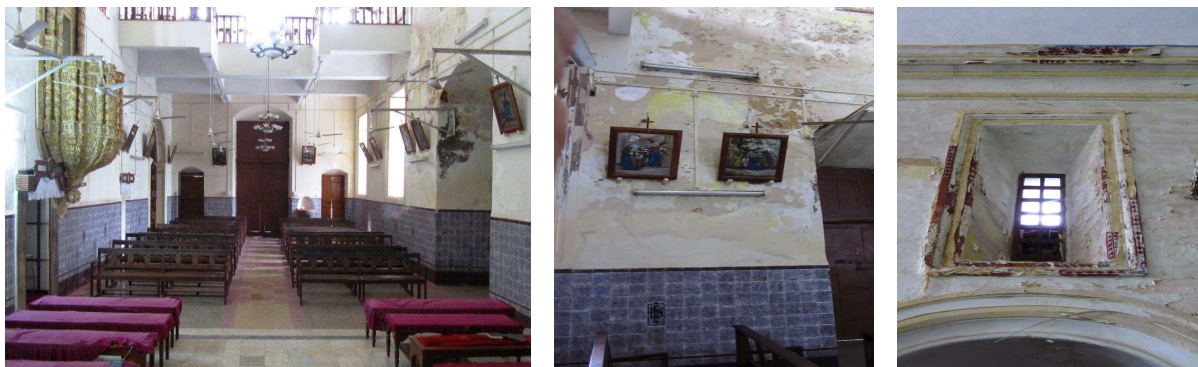
Figure 5: Conflict of materials and damage on the surface of the inner walls of the nave.
