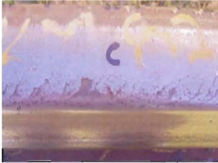
Figure 1.7: Rail head check, [8].
