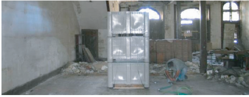
Figure 13. Load test on a timber floor. António Carneiro building, XX century (1916), Porto.
