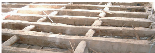
Figure 4. Beams and transversal bars of a timber floor. São Domingos building, XIX century (1856), Porto.
