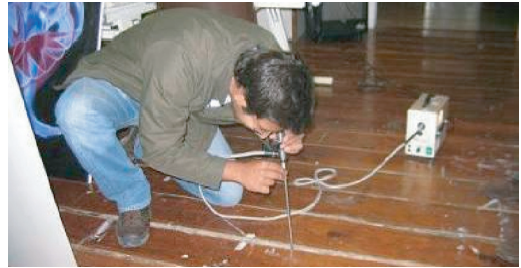
Figure 8. Use of the videoscope for the visualization of a timber floor. Belomonte Palace, XVIII century, Porto.
