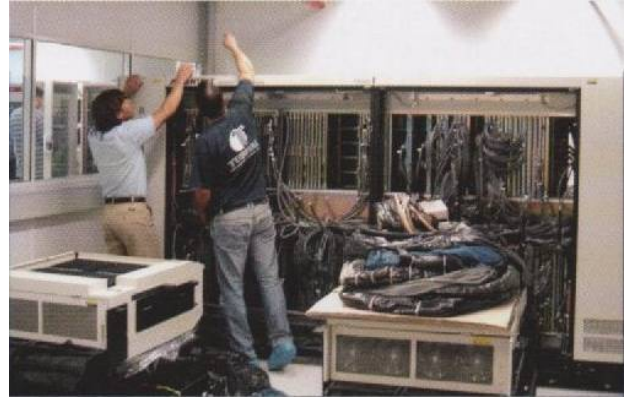
Figure 2: T5365 installation and set up at Qimonda.
