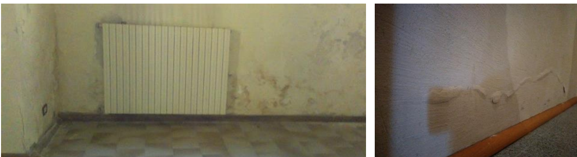
Fig 4.6 – Plaster detachments on a wall from the ground floor (left); Lower part of wall from the conference room (right);
