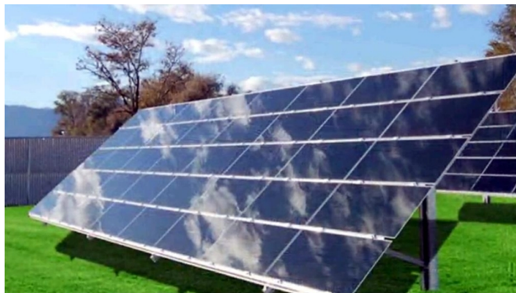
Fig. 1.5 Photograph of park of thin film solar cell panels, (CNET, 2010)
