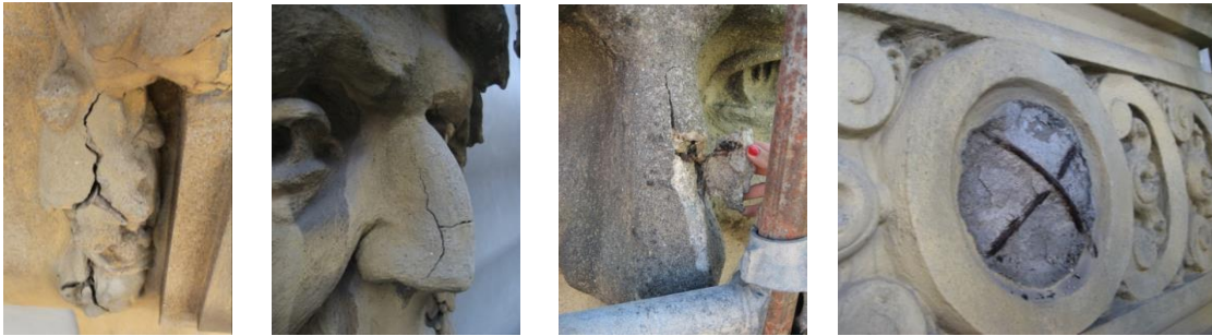
Figure 1 – Examples of reinforced concrete decorative elements and sculptures exhibiting some level of material degradation.
