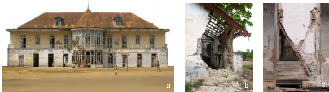
Figure 11. Example of the built heritage within the estates and their advanced state of degradation, Roça Boa Entrada, São Tomé – (a) main house, (b) warehouse, (c) technicians' house [ASF+HMS].
