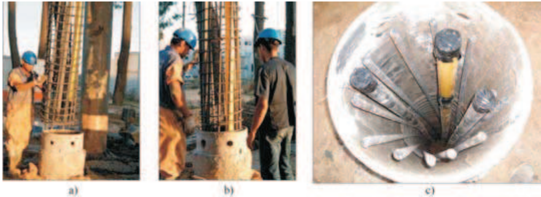
Figure 10 - a) and b) Reinforcement installation; c) Final positioning of the reinforcement (Costa Esteves, 2005).
