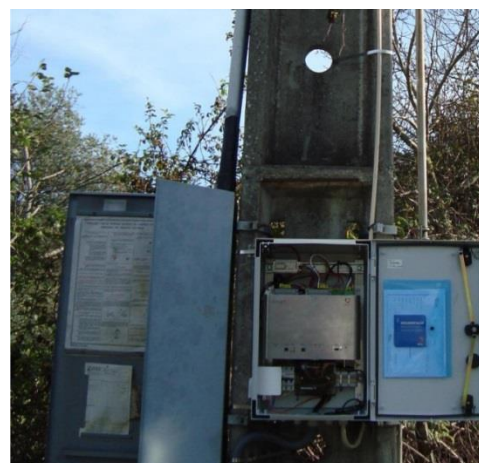
Figure 1 - Example of DTC installed in Pole MVS
