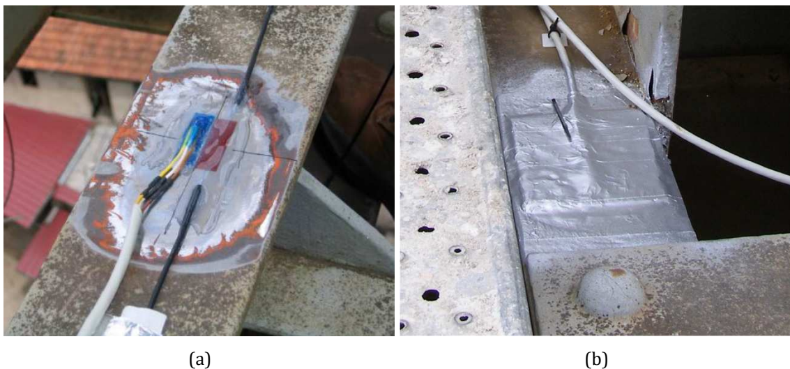
Figure 2.5 - Sensors installation: (a) strain sensors ES6-1 and OS6-1 in section S6 during the gluing process; (b) final aspect for sensor ES9-1 in section S9.
