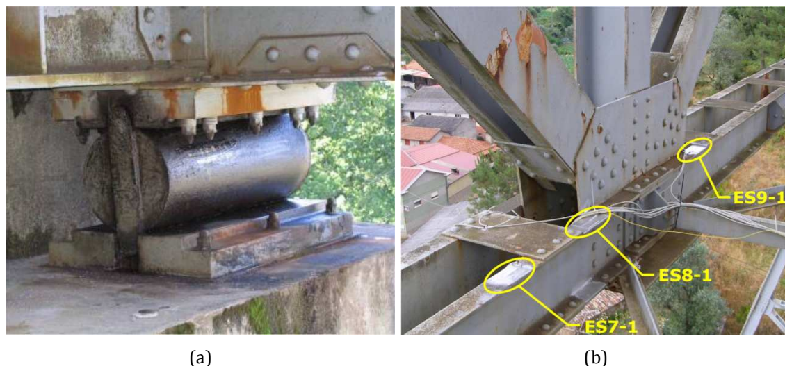
Figure 2.2 - Details of the bridge structure: (a) bearing placed at the west abutment; (b) lower joint of the truss girder instrumented with strain sensors in its vicinity.
