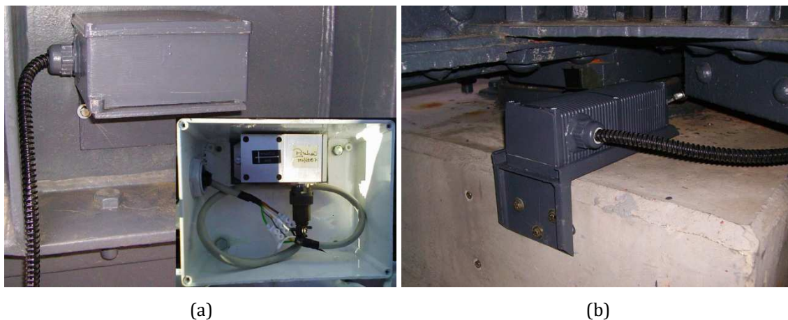
Figure 3.10 - Protection systems applied to sensors: (a) inclinometers; (b) displacement transducers.
