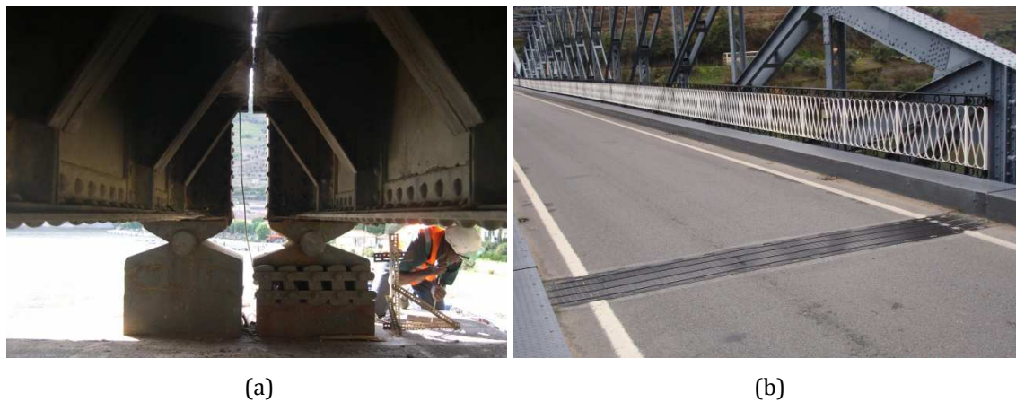
Figure 5.16 - Expansion joint: (a) bottom view before the rehabilitation; (b) top view after the rehabilitation.
