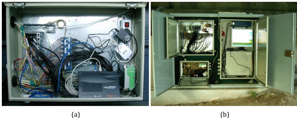
Figure 3.11 - Observation stations of the monitoring system: (a) Observation Station (OS); (b) Central Observation Station (COS).
