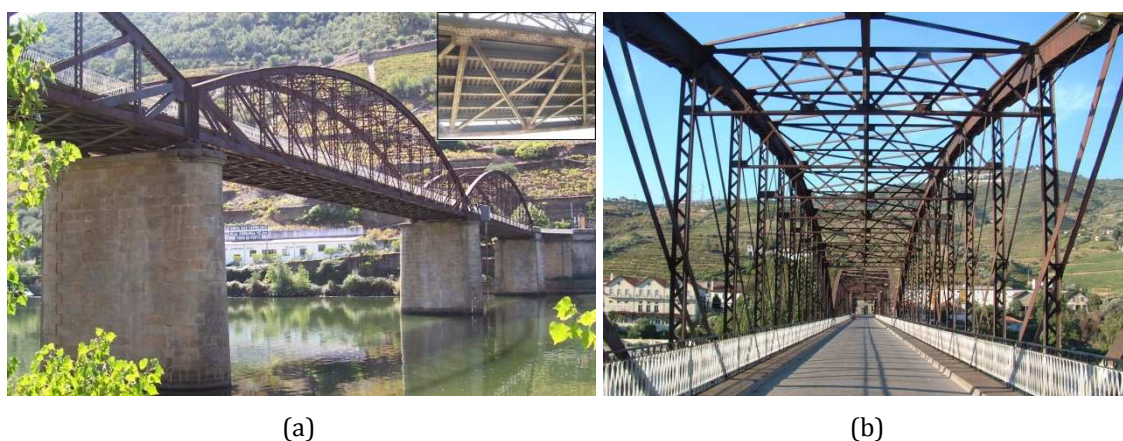
Figure 3.4 - Pinhão Bridge before the rehabilitation: (a) side and bottom views; (b) view from the road (inner view).
