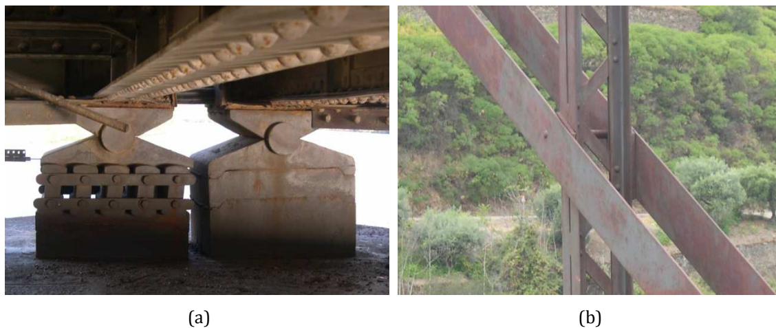
Figure 3.3 - Pinhão Bridge before the rehabilitation: (a) roller (left) and pin (right) bearings; (b) intersection node of a diagonal with a vertical.
