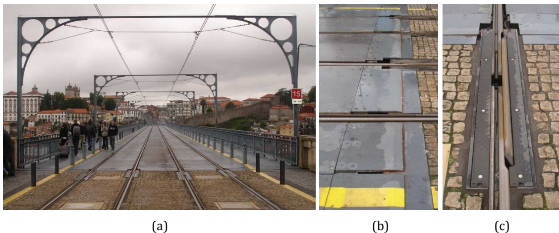
Figure 8.8 - South abutment of the upper deck in the new service phase: (a) general view; (b) cover plates of the expansion joint; (c) expansion device of a rail.
