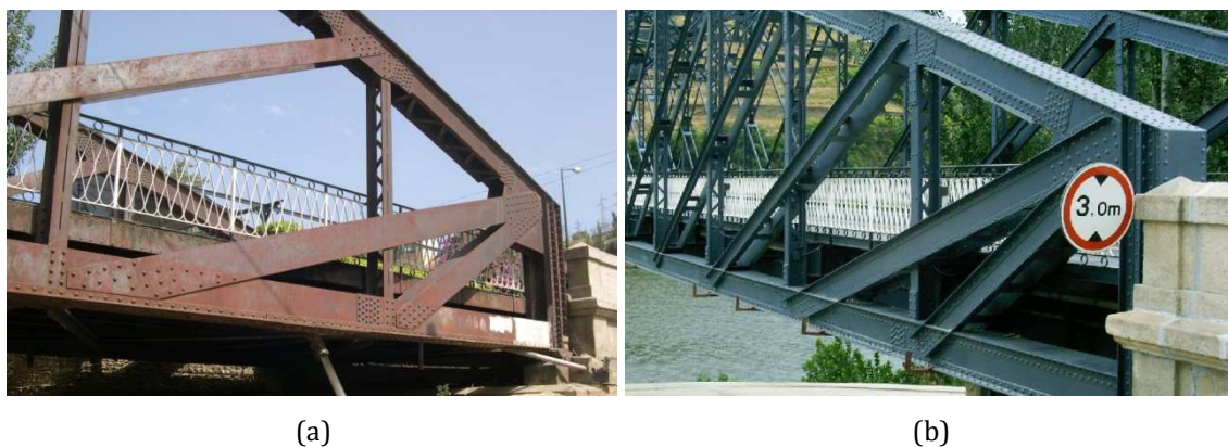
Figure 5.10 - Diagonals of the truss girders: (a) before the rehabilitation; (b) after the rehabilitation.
