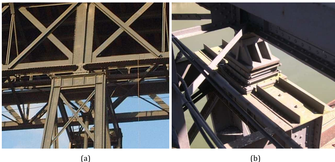
Figure 7.25 - Load transfer from the upper deck to piers P1, P2 and P3: (a) side view of the top of pier P2 after the rehabilitation process; (b) view of the upstream bearing located at the top of pier P1 (picture taken from the technical path of the upper deck).
