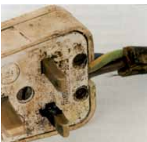
Damaged cable grip
