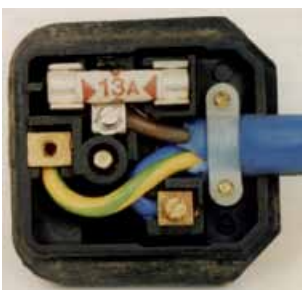
Missing screw on earth connection
