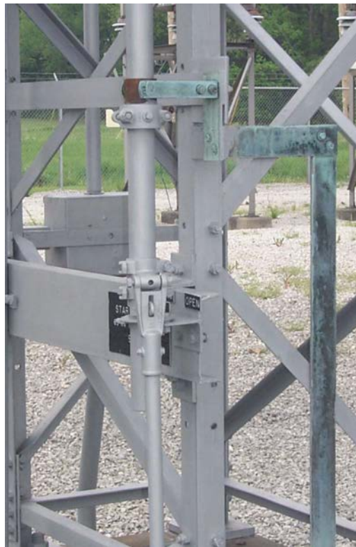
Figure 36—Typical braidless grounding device
