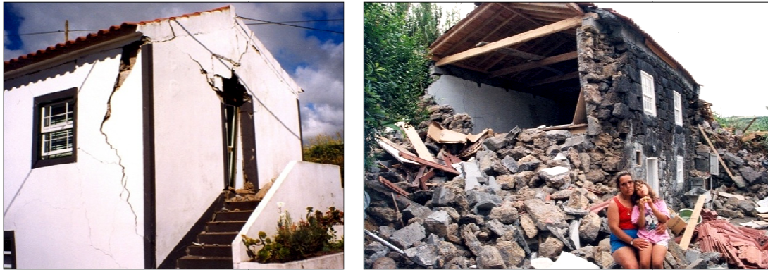
Figure 4.2. Damage and collapse of the gable and transversal wall, Azores 1998 earthquake
