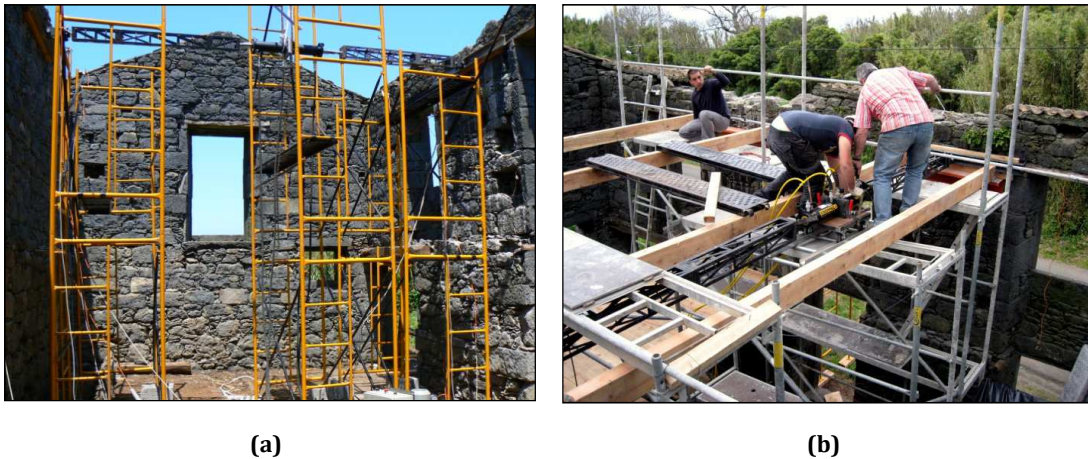
Figure 3.1. In-situ actuation system for the tested building: a) CS_01 test; b) preparation of the CS_02R test
