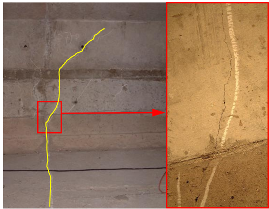
(b) Crack detail at section n°21
