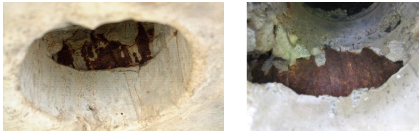
Figure 7.9 – Prestressing ducts exposed at the bottom slab.
