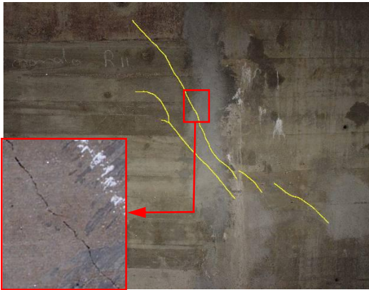
(c) Crack detail at section n° 55.
