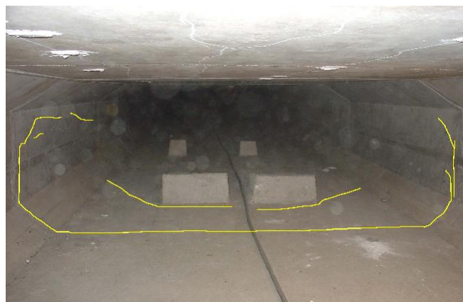
(c) Detail of the crack development at section n°23.
