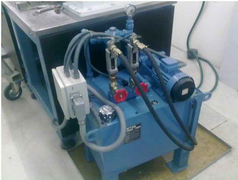
Figure 3.2.: Hydraulic oil supply station.
