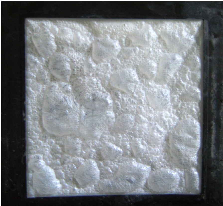
Figure 2.15 – View of a blistered membrane.
