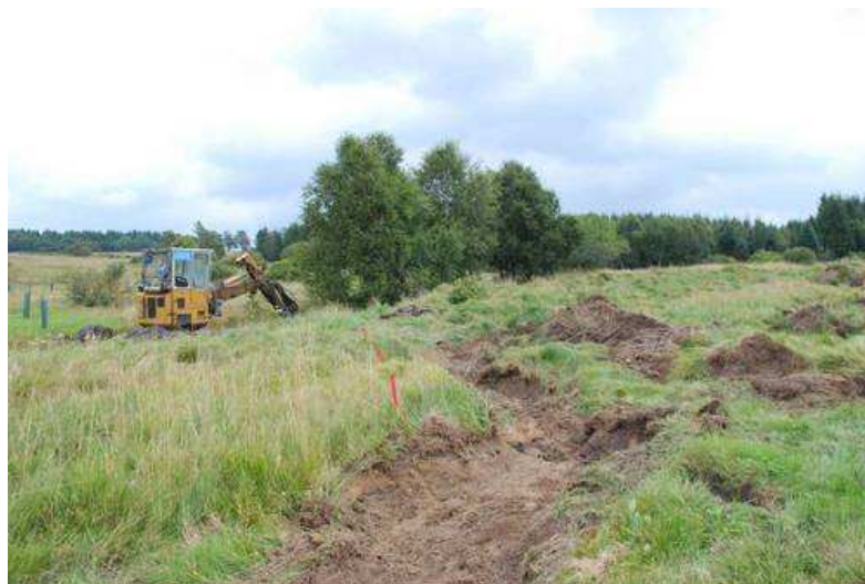
Fig. 21: Machinery opening meanders in the upper part of the stream (by ANCLP CR)
