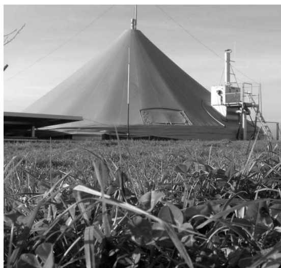
Figure 4.13 – Biogas storage system in Burgenland, Austria
