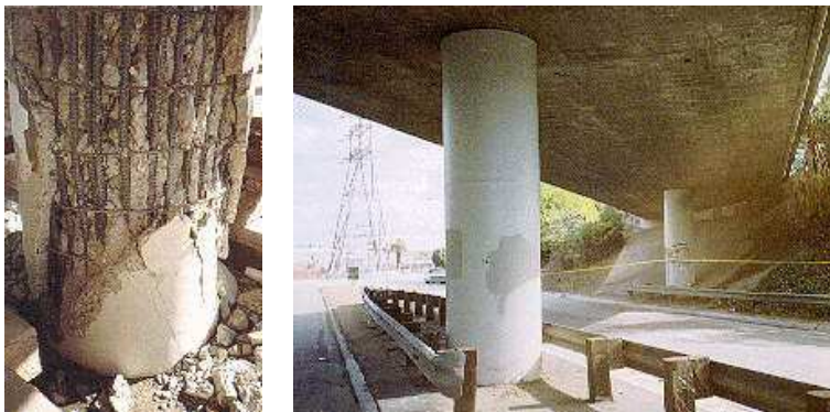
Figure 2.6 – Failure of column due to failure of circular confinement steel ( left ); good behaviour of column retrofitted with steel jackets ( right ).
