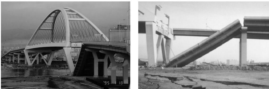
Figure 2.9 – Nishinomiya-ko Bridge approach span collapse (Kobe Collection, EERC Library, University of California, Berkeley).
