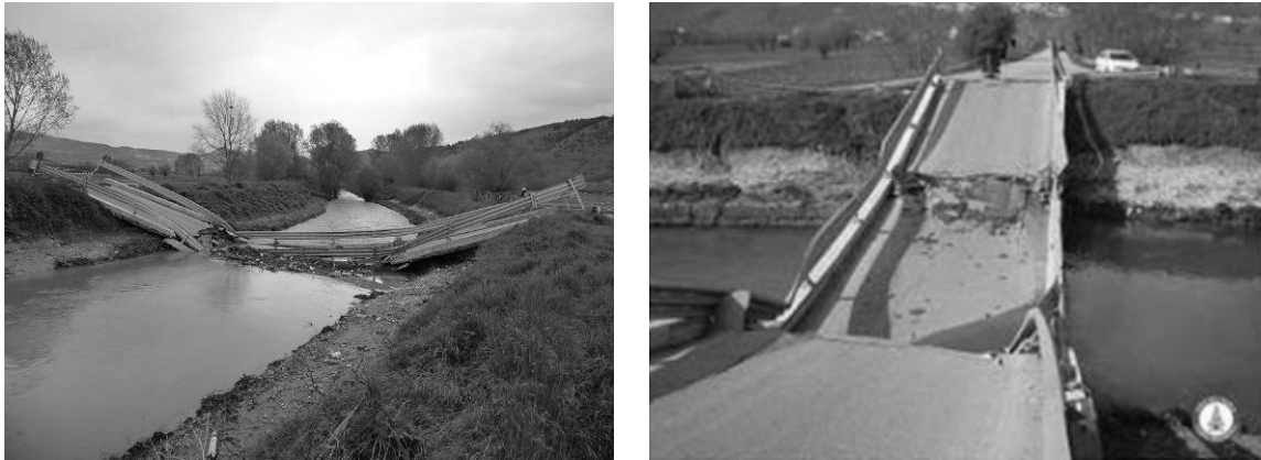
Figure 2.10 – Bridge collapsed on the Aterno river, near Fossa (Grimaz and Maiolo, 2010).
