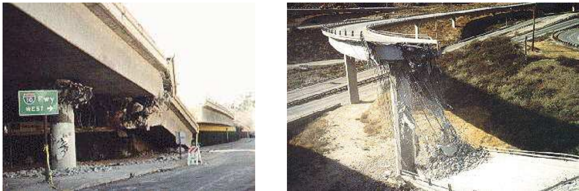
Figure 2.4 – Collapsed sections in Santa Monica freeway ( left ) and Antelope Valley Freeway ( right ).
