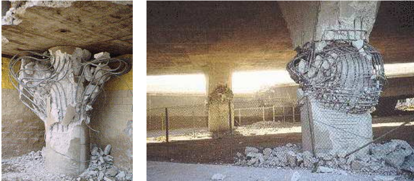
Figure 2.5 – Failure of columns: insufficient confinement ( left ); shear failure of flared column with transverse reinforcement slipping ( right ).
