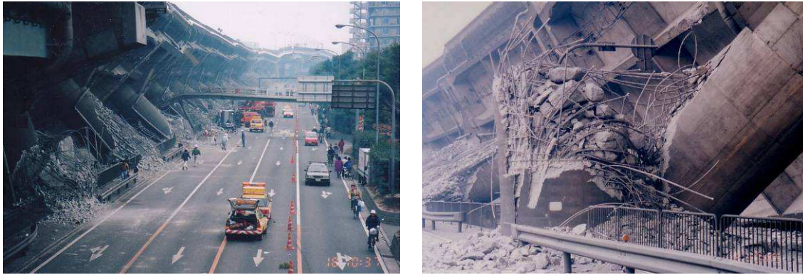
Figure 2.7 – Collapsed Fukae Viaduct ( left ) and Premature Shear Failure of Reinforced Concrete Column, Fukae Viaduct ( right ) (Kawashima, 2007).
