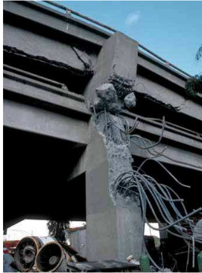
Figure 2.2 – Cypress viaduct: lack of proper reinforcement in pier-deck connections.
