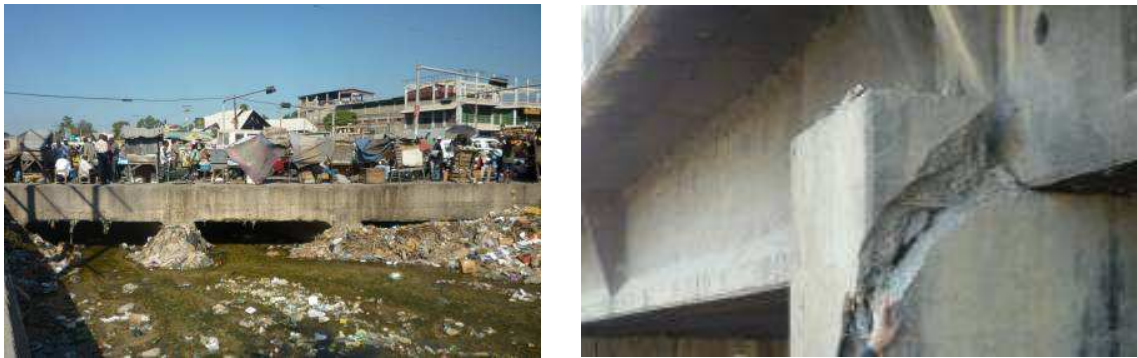
Figure 2.11 – Box culvert in Port-au-Prince ( left ); damage to shear key at intermediate support of bridge ( right ) (Eberhard et al. , 2010).
