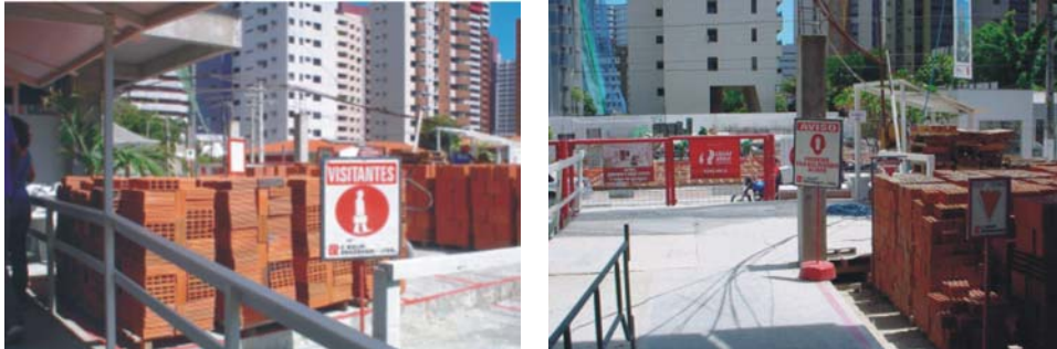
Figure 14 – Fixed storage area (left) and pathway (right) seen from an open wooden tunnel at a construction site in Fortaleza. Source: Miranda Filho (2008)
