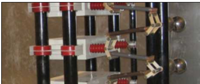
Figure 3.8 - Detail of the generator stack.
