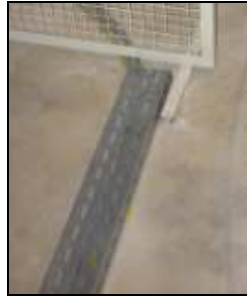
Figure 8.6 - Metallic gutter which protects electrical cables.
