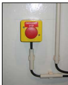
Figure 8.5 - Emergency stop switch of the High Voltage Laboratory.
