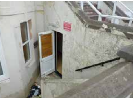
Figure 1 – once grand but now poor condition housing
