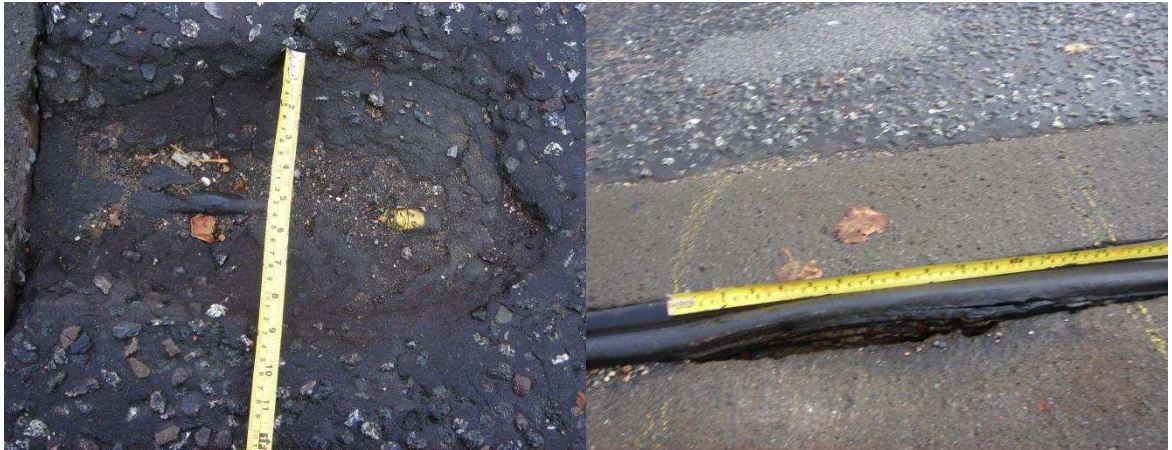
(a) – Asphalt potholes with visible rebar on Span 3 (b) –Expansion joint between span 3 and 4
