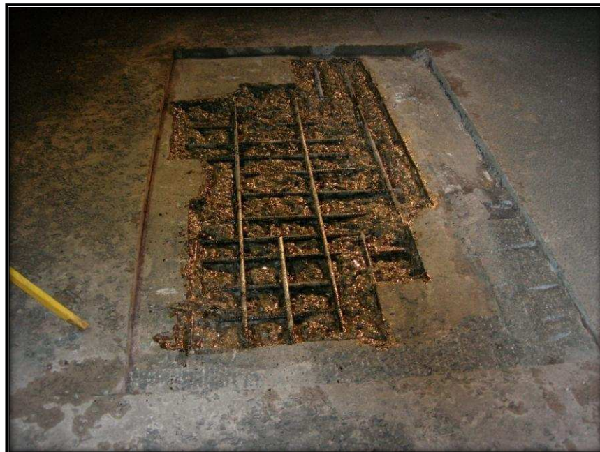
Figure 4.8 – Area 1 of visible rebar (Photo from Kevin Banks, 2010)
