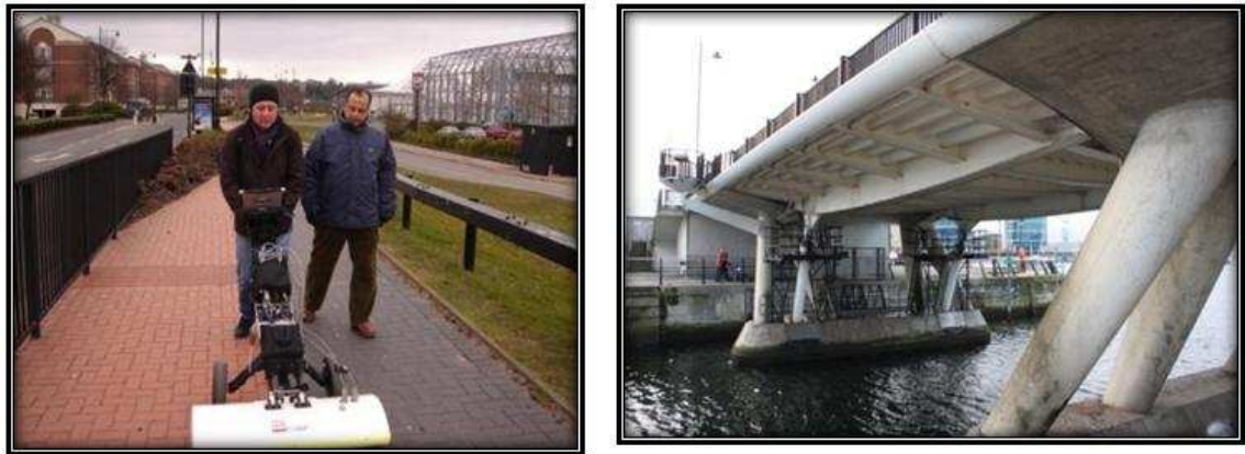
Figure 4.11 – GPR Survey on the St Marys Island Lifting Bridge. (photo from Gokhan Kilic, 2010)
