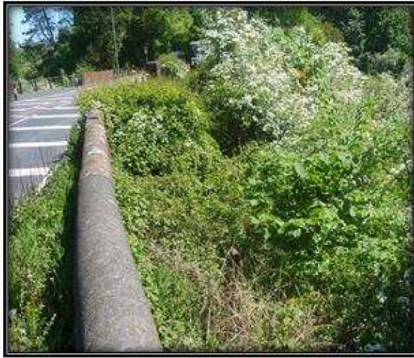
Figure 4.16 – Heavy vegetation North side view of the bridge (photo taken by Gokhan Kilic, 2010)
