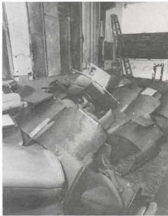
The chairs are amongst the many materials being upgraded in the Bakst Auditorium renovation.
