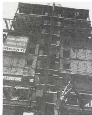
The new research building is rapidly losing its skeletal look, as concrete and brick are applied to the exterior of the building.
