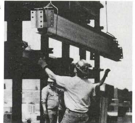
Iron workers on the site of the Center for Advanced Biomedical Research guide a steel beam as a crane lifts it into the air.
