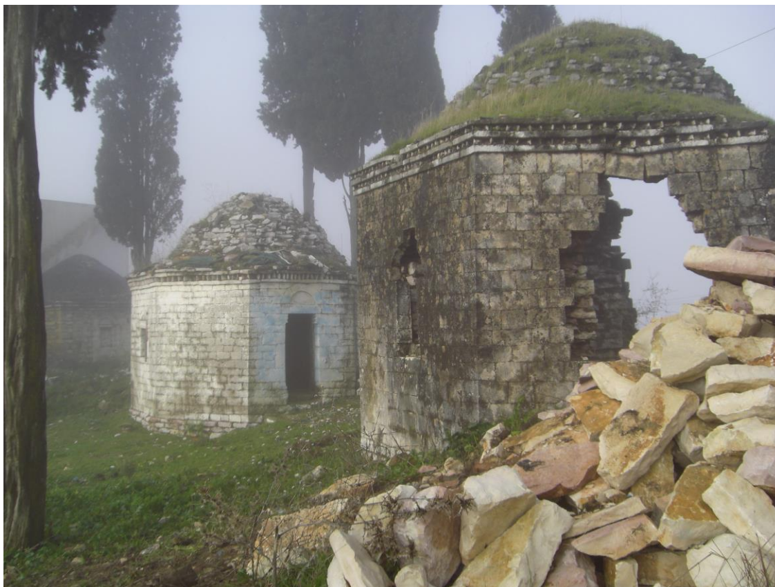
Figure 3.3. Bektashi shrines showing signs of neglect and awaiting repairs. Gjirokastrë, 2007.
