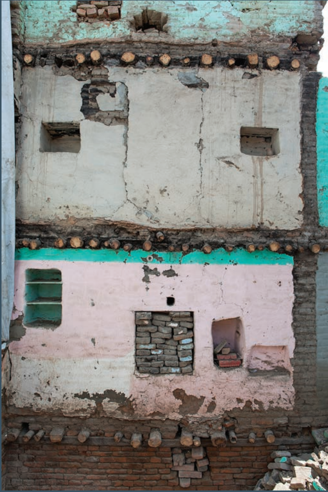
In a neighborhood on the east side of Bhaktapur, interior walls of family houses were exposed by the collapse of roofs and neighboring buildings.
