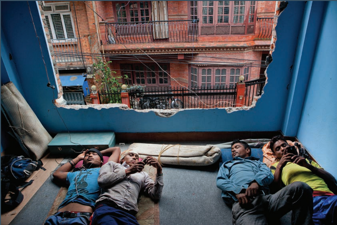
At mid-morning, laborers in Kathmandu's Naya Bazaar take a break from their heavy work tearing down buildings. These four young men came to Kathmandu looking for work after the earthquakes. They lived in the building that they were tearing down with eight other friends from villages in the southeastern Udayapur district. These workers, numbering in the several thousands across Kathmandu and other affected areas, were paid by the owners of the properties that they deconstructed.
