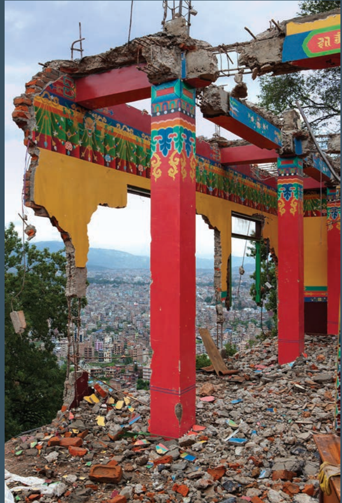
By mid-June 2015 there was little left of the Karma Raja Maha Vihara monastery on the Swayambunath hill, west of downtown Kathmandu. The monastery was badly cracked and was taken down under the supervision of UNESCO and the Karmapa ShaMarNag Committee.
