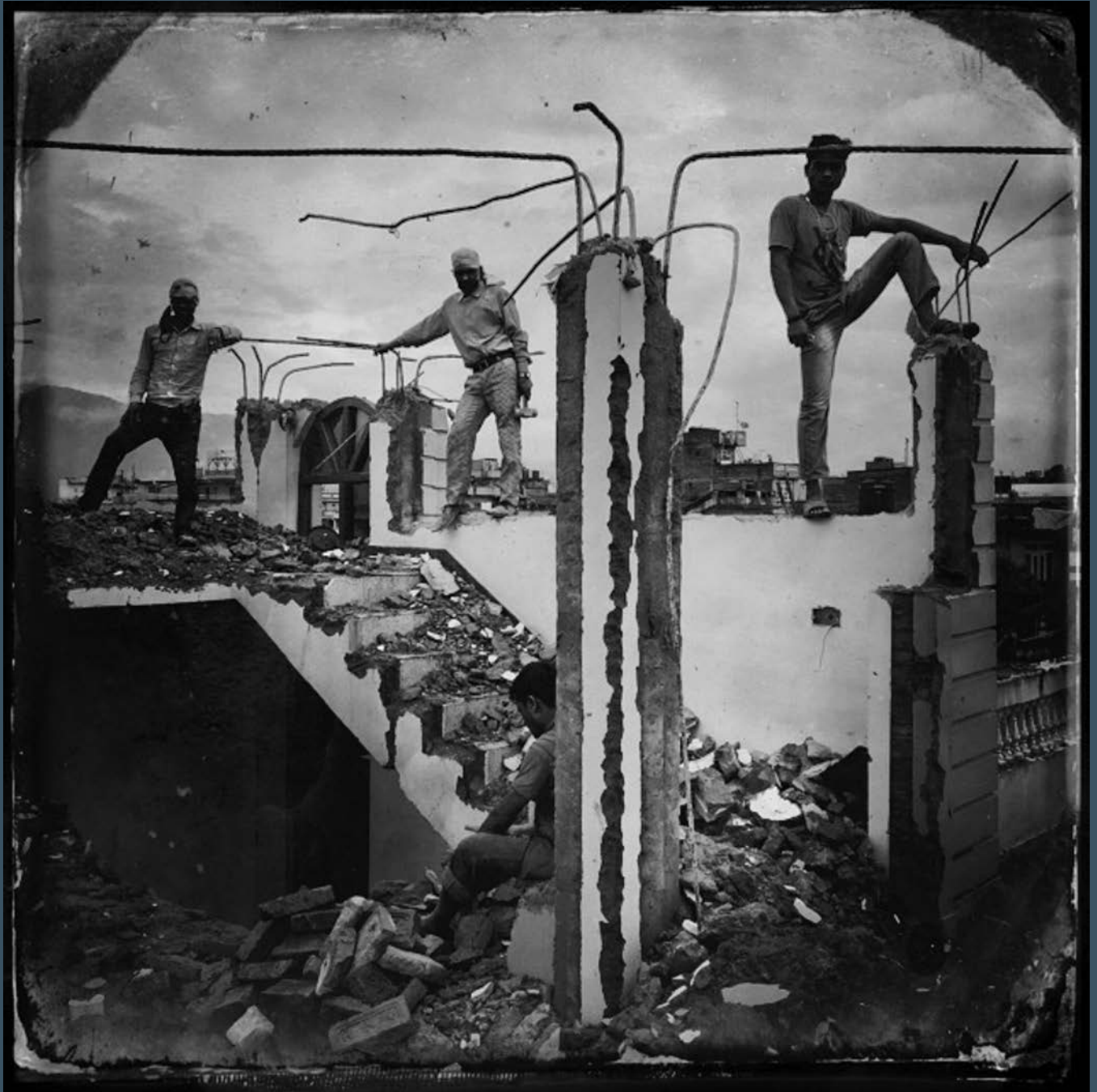
Demolition of concrete buildings continued through monsoon season downpours. Balaju, Kathmandu, Nepal.
