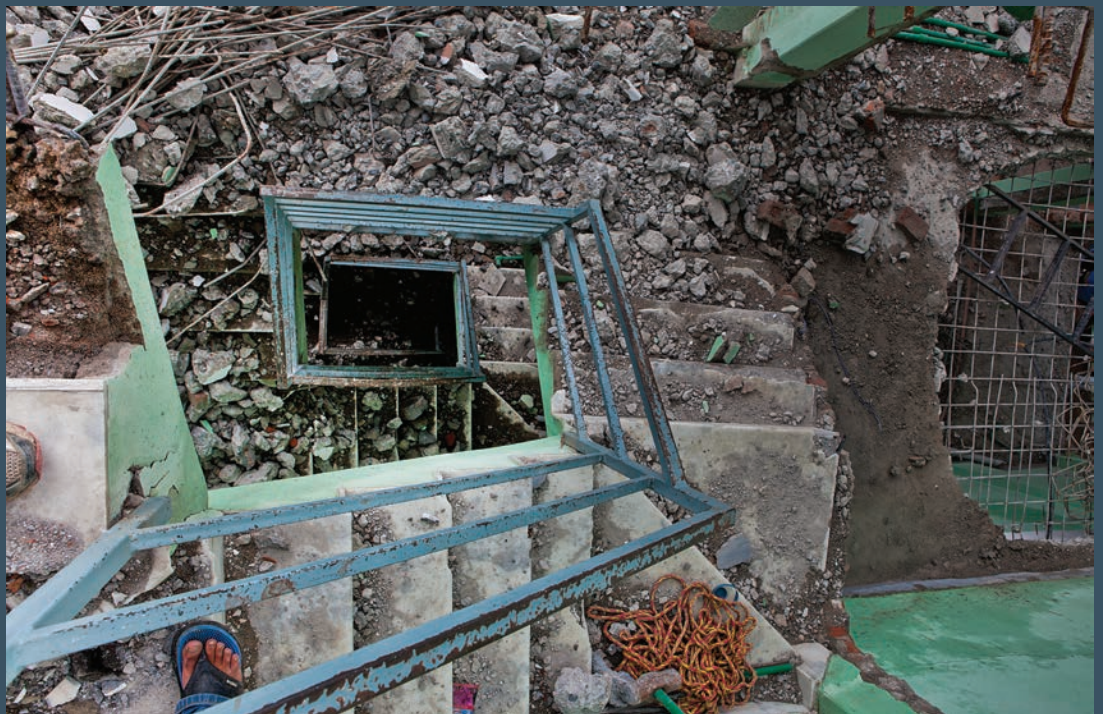
The fourth-floor stairway of a building under demolition is covered in rubble. Such stairways became internal chutes for rubble to be brought down to ground level. Workers made holes by pick axing and hammering through concrete and rebar floors in order to let rubble fall down to the lower levels. This way, the demolition laborers did not have to carry heavy loads of debris down the stairs.
