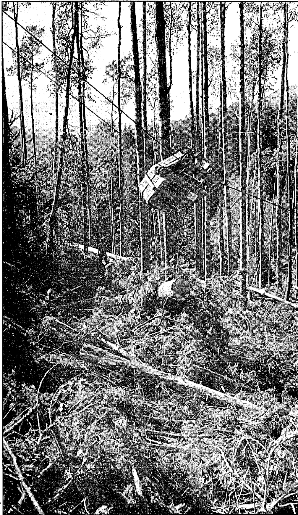
KEN BARNARD'S cable log hauling system was one of three locations recently visited by a Caledonia forestry science class. Arranged with the help of Forest Renewal B.C., the tour gave the students insight into different kinds of logging and of the importance of restoring and keeping habitat for animals and fish.
