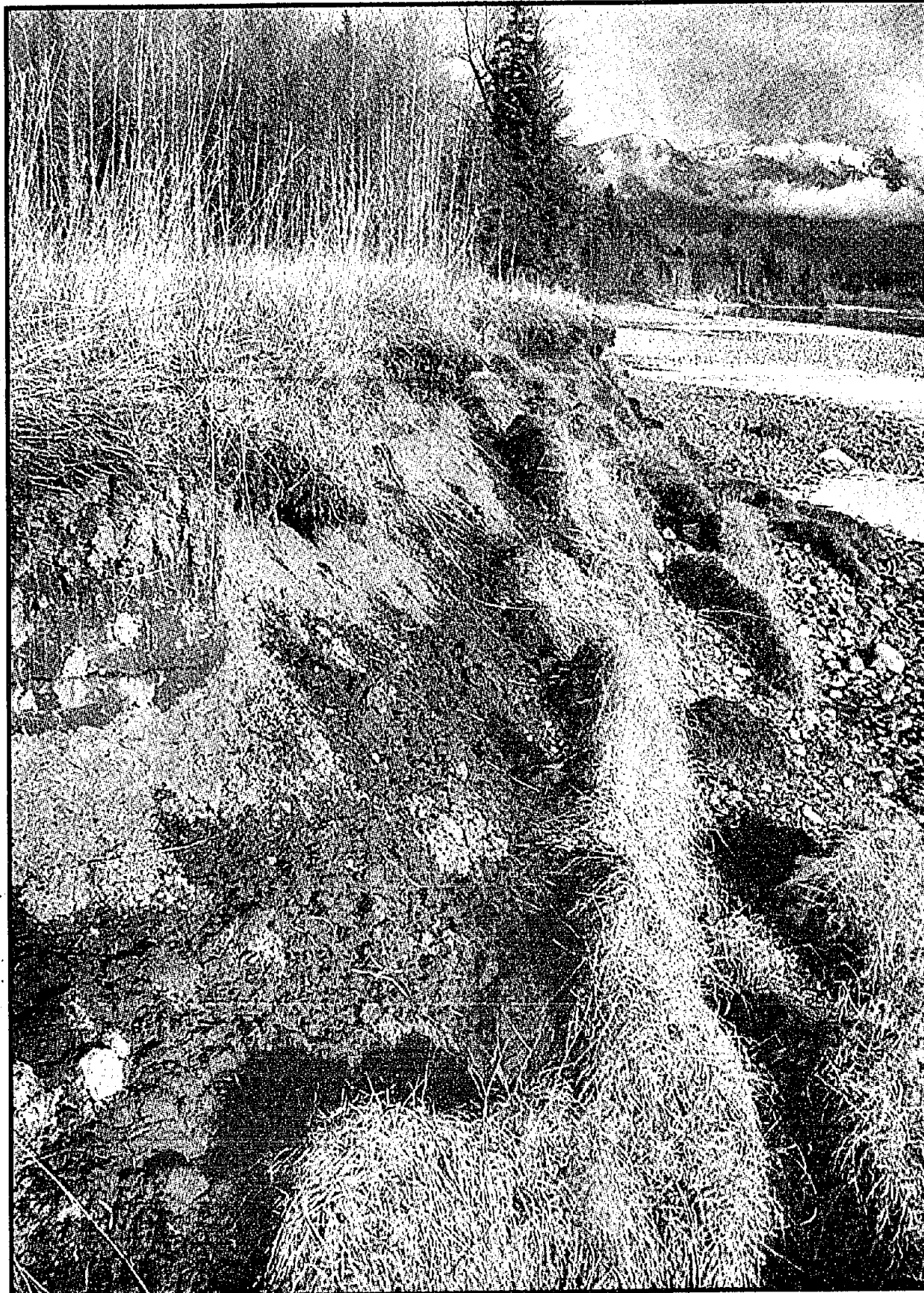
GOING, GOING, GONE: The bank of the Skeena River is eroding dramatically just a stone's throw from the city's sewage treatment plant. City officials estimate they'll have to spend at least $1 million rip-rapping the bank in future years to keep the river from punching through to the lagoons. JEFF NAGEL PHOTO
