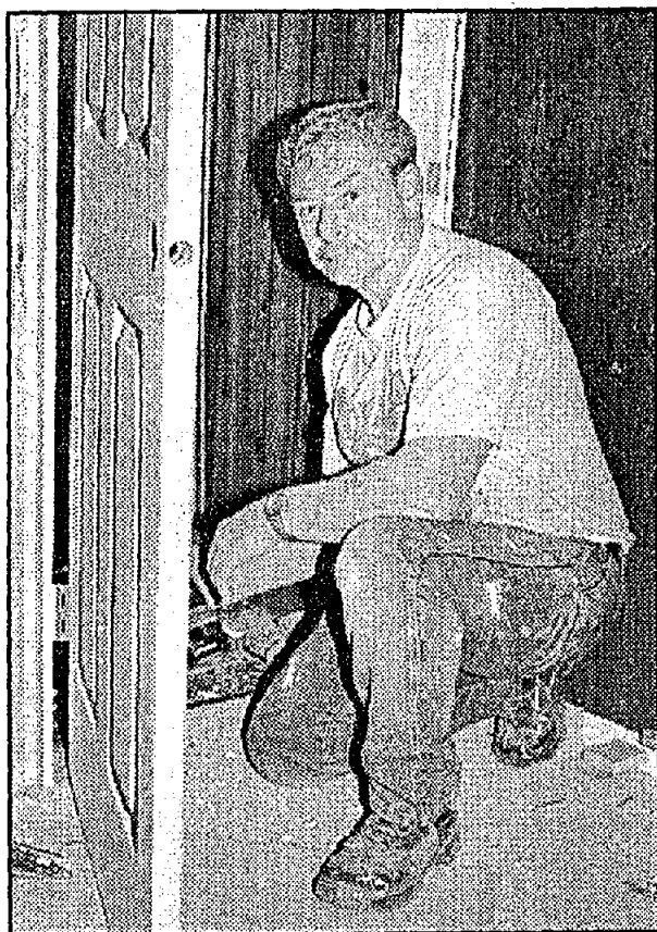
A HOUSE on Queensway has been purchased by an arm of the Nisga'a Lisims Government as a residence for foster children. That's Harley Chisholm of S.W.H. Masonry and Construction working on some of the renovations.
