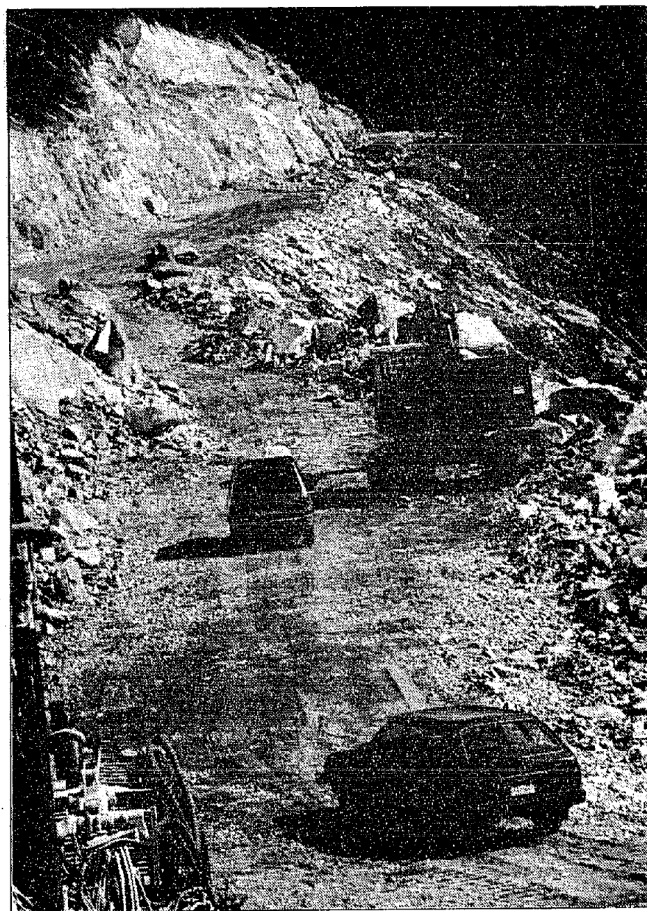
The Ministry of Highways and local sub-contractors spent this summer and fall upgrading the last 5 km of the Shames Mountain Access Road to a Highways standard 50 - 70 km speed road.
