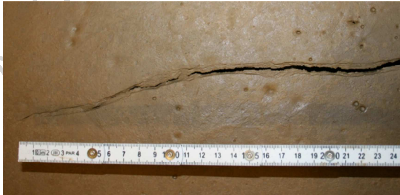
Figure 5: Surface depression on the clay surface ahead of a crack.
