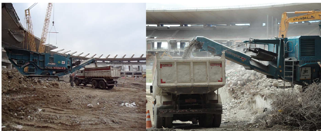
Figure 1. The recycling process of the construction waste on site, done by a crusher machine
