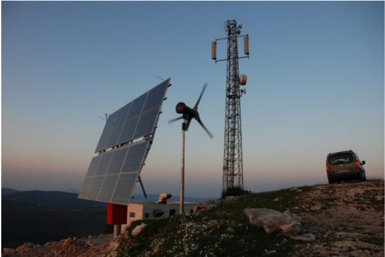
Fig. 1.5 solar- and wind-powered base station at Villarceaux [24]
