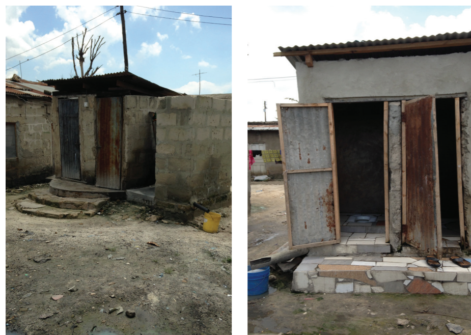
Structural conditions of the toilets in Mlalakua Ward. Source: Author
