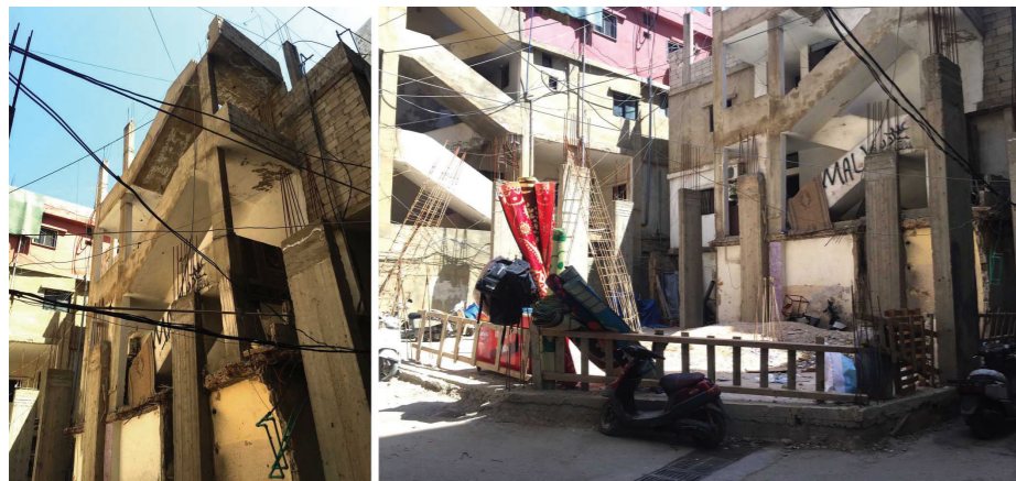
Fig.14) The chaotic structural systems (left). Foundation of new buildings start from above ground (right).
